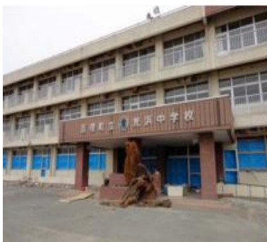
The doors and windows were broken by tsunami on 1 st floor
